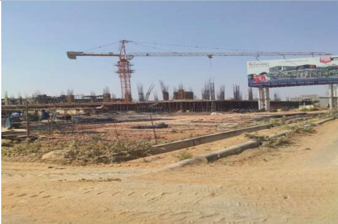
Picture6: Tower Cranes
